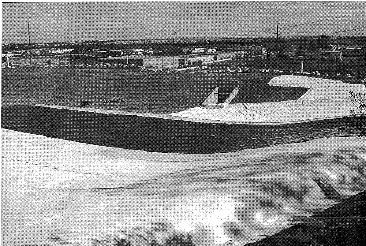
Fig. 6. Photograph taken during installation of the upper storm water pond liner showing placement of VFPE geomembrane (black) over GCL (white). Note white landfill gas vents along the crest of the pond berm.
